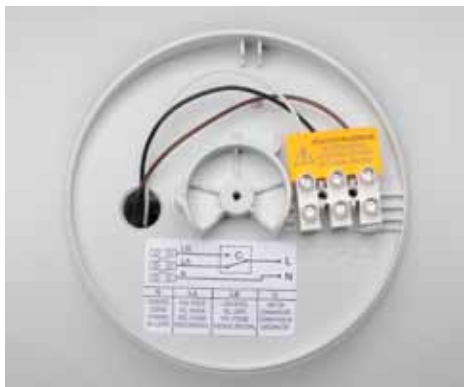
Connect electrical supply.
