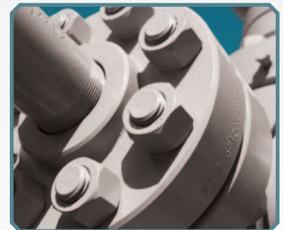
Bolts and edges
