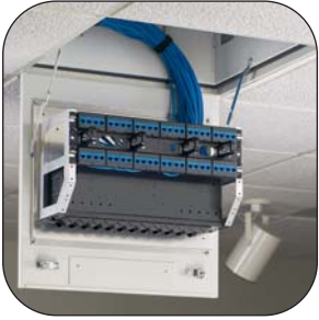
Zone Cable Boxes
