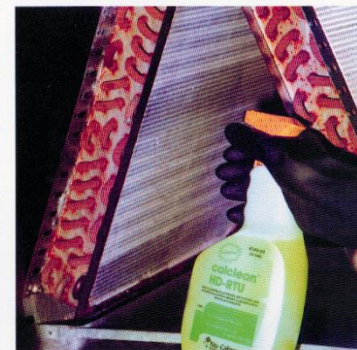
Coil cleaning is one of the most profitable service procedures a contractor can offer.
