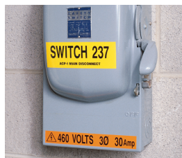
Panel & Switch ID
