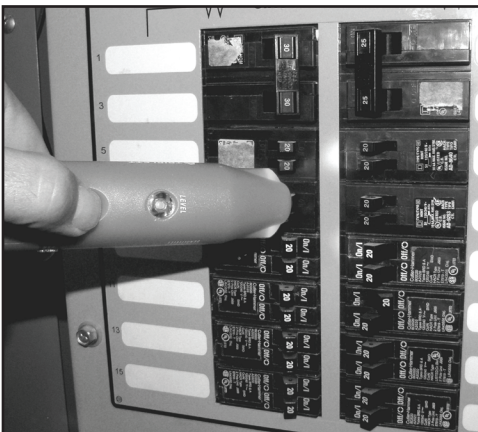
Identifying breaker by locating the "null".
