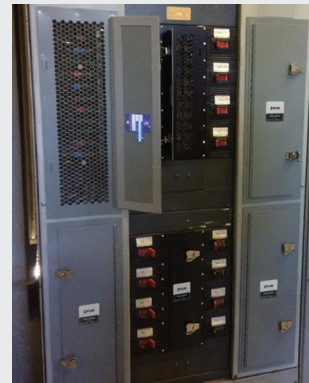
Figure 2: 24-inch IR window installed at SLAC
