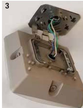
Complete wiring connections.
