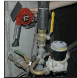
Thaw Frozen Pipes
