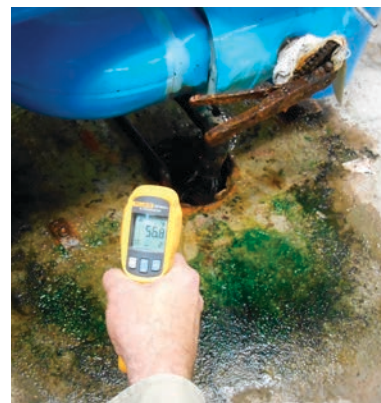
Taking the temperature of condensate as it goes into the drain.
